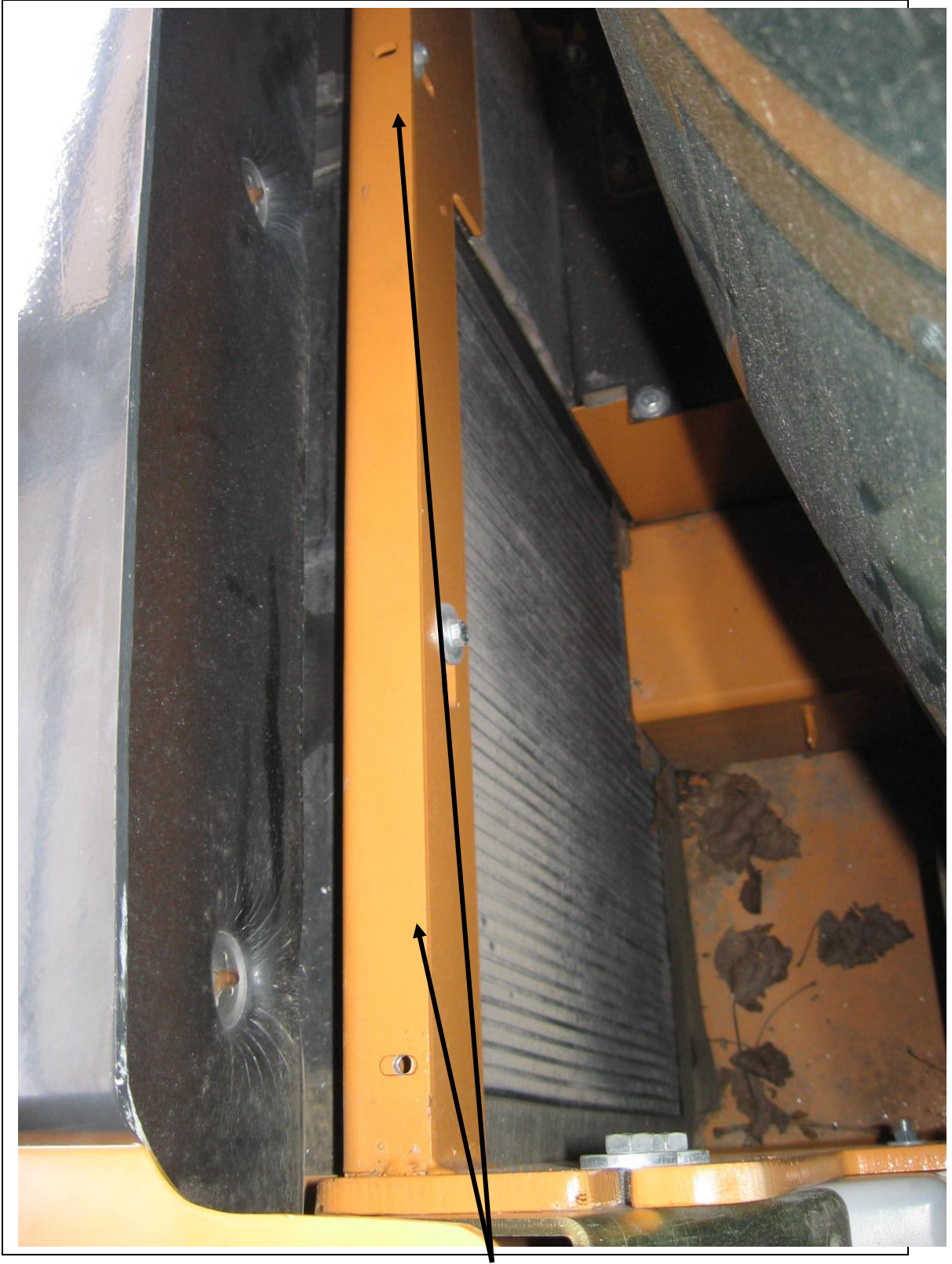
Condenser mounts here.
